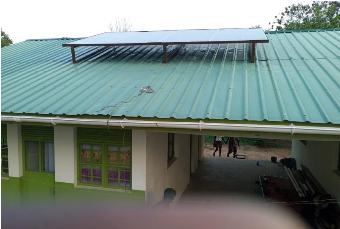
Figure 12-Solar Installation in Atil camp
